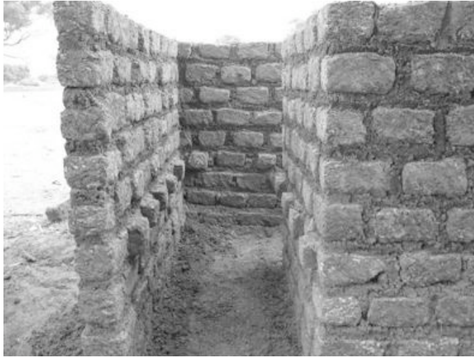
Figure 6.10 The entranceway of a latrine made from laterite brick and clay mortar. Note the protruding bricks (placed sideways) which provide handhold support for latrine users.
