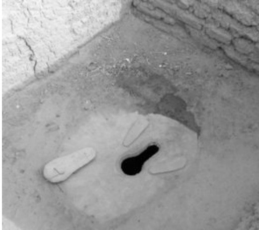
Figure 6.3 A sanplat latrine soiled by urine from improper use and poor drainage.
